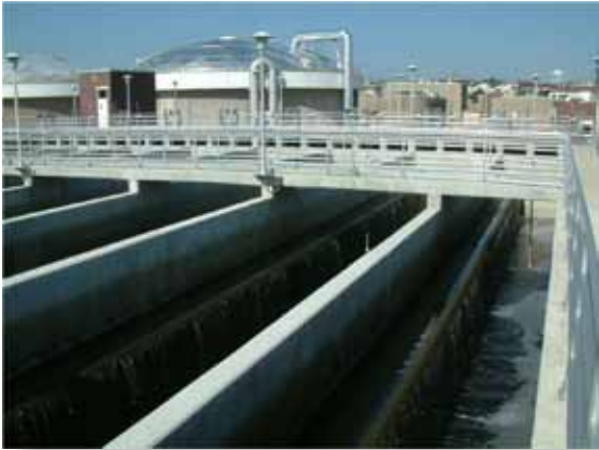
Littleton Englewood - Tetra® Denite® Filter System
