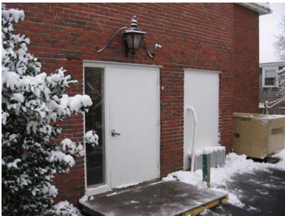
Wastewater treatment plant control room containing control panels and MicroC™ storage. The plant is located sub-surface beneath parking lot (see reverse for schematic).
