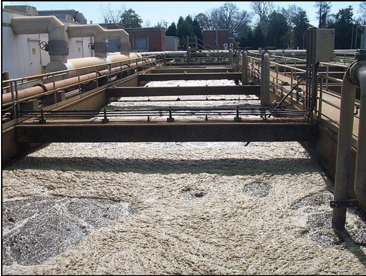
This demonstration train at HRSD James River Treatment Plant was reconfigured for testing purposes.
